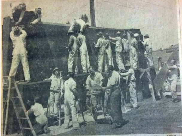
CARPENTRY WORK on Burlingame's Honor Roll nears completion on the Park Road lawn of the post office as more than 30 volunteers aided in the construction last Sunday morning. Shown in front of the roll, consulting plans, are left to right, U. S. Simonds Jr., business agent of Carpenters Local 162 and chairman of the construction committee; William Feary, member of the construction committee, and George McQueen, who serves on the general committee of which Emil Schultz is chairman. Plastering work on the roll is expected to be done this weekend and work has started on painting the names of the servicemen and women on the panels. (Photo by Anita Fowler).
