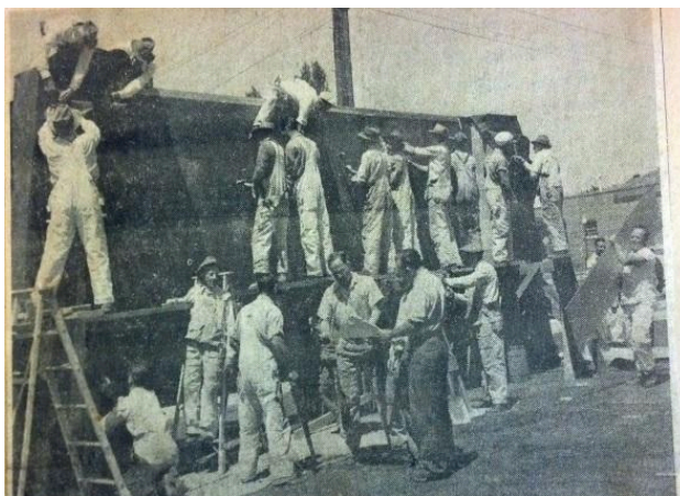
CARPENTRY WORK on Burlingame's Honor Roll nears completion on the Park Road lawn of the post office as more than 30 volunteers aided in the construction last Sunday morning. Shown in front of the roll, consulting plans, are left to right, U. S. Simonds Jr., business agent of Carpenters Local 162 and chairman of the construction committee; William Feary, member of the construction committee, and George McQueen, who serves on the general committee of which Emil Schulz is chairman. Plastering work on the roll is expected to be done this weekend and work has started on painting the names of the servicemen and women on the panels. (Photo by Anita Fowler) Burlingame Advance 6/14/45
